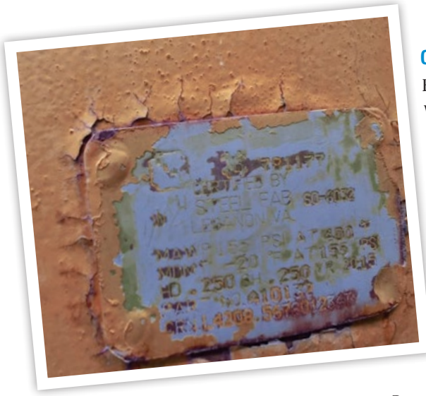
Compressed air storage tank identification plates advise when the last safety inspection took place.
