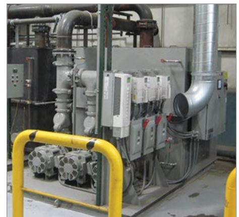
Typical standalone control system with on-skid pressure sensing and pump VFDs.
