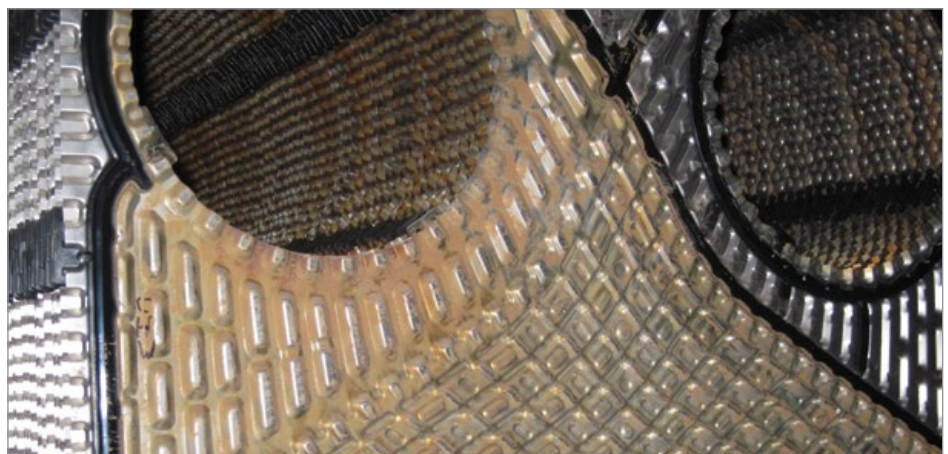
Sediment on the open loop side of an isolation plate heat exchanger before cleaning. This material was kept out of the plant machine heat exchangers.
