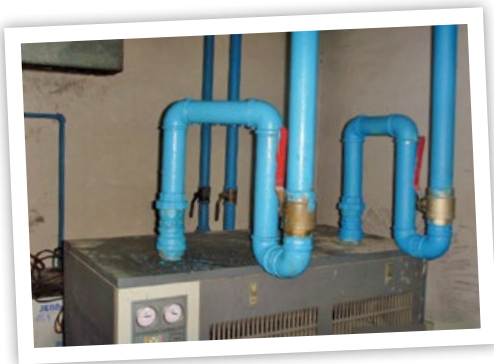
The U-turns in the steel piping leading to this refrigerated compressed air dryer cause pressure drop.
