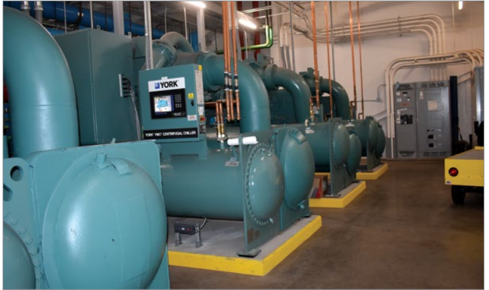
Two YMC ® and 2YKs chillers provide the needed cooling for both comfort and process.
