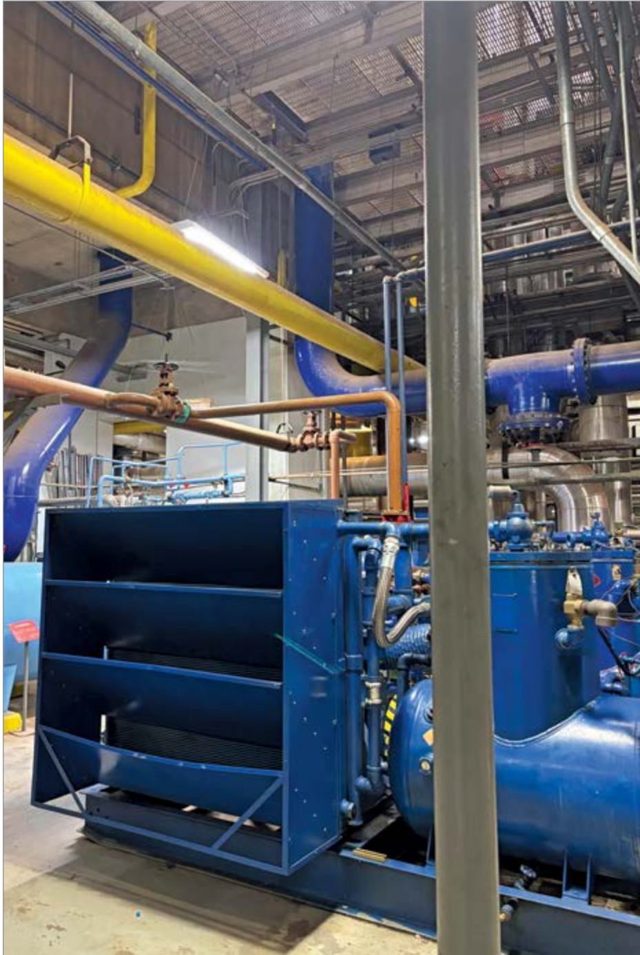
The Texas university's disassembled 300 hp air compressor was reassembled at this location, replacing an older 300 hp air compressor.
