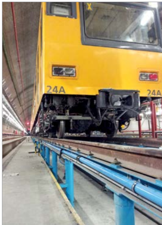
The maintenance shop for this light rail line is powered by compressed air delivered through modular aluminum piping. (Courtesy of Parker-Transair.)
