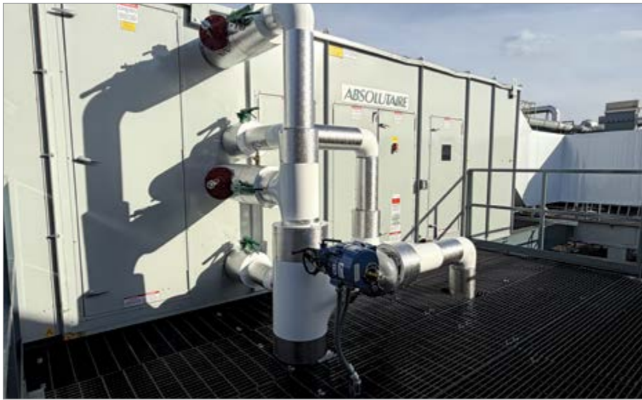
An exterior piping connection allows the make-up air unit coils to use the recovered energy.
