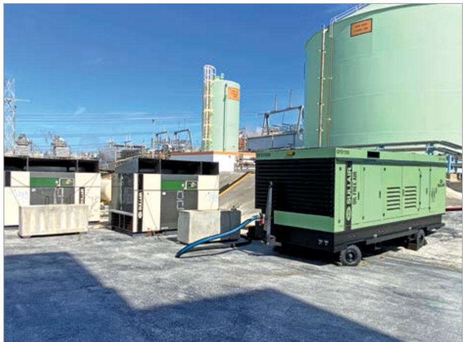
A major utility runs this oil-free portable air compressor and the two older oil-free rotary screw air compressors behind it.
