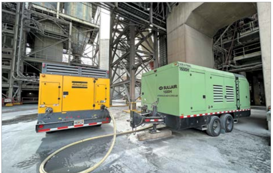
These portable diesel air compressors are used in a cement plant.
