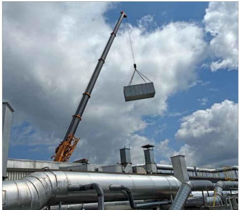
Coordinated rigging and crane work was essential to set and assemble the makeup air unit.
