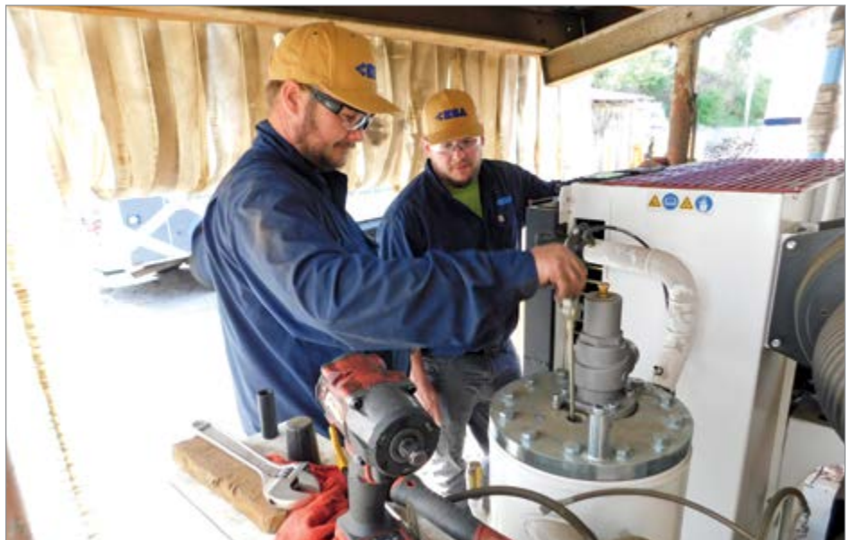
A technician performs an oil separator element changeout on an oil-flooded, rotary screw air compressor as part of a scheduled preventive maintenance service.
