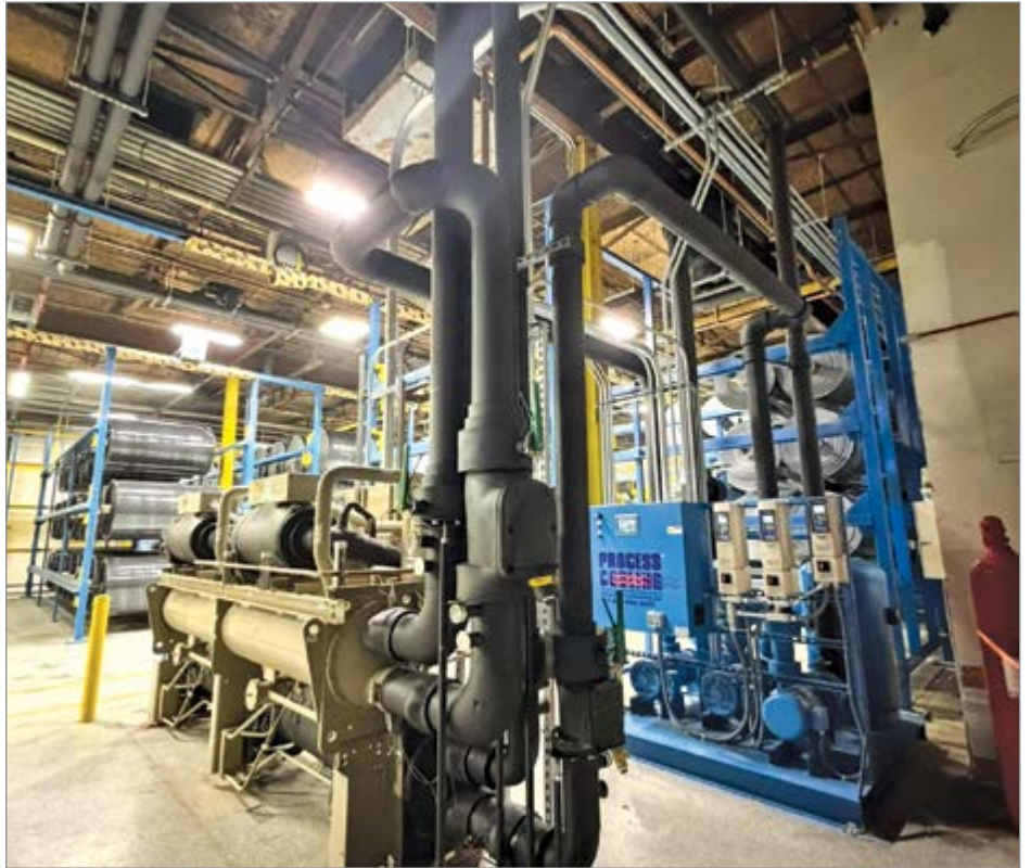
A central heat recovery equipment circulates fluid between the house chilled water system and the recovery system.
