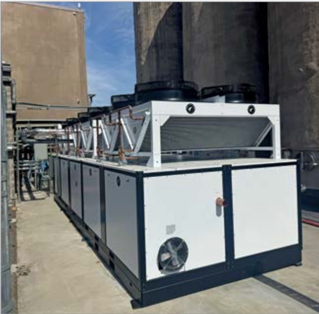
A six refrigeration compressor, propane refrigerant chiller with an oversized air-cooled condenser installed at Waterbrook Winery.
