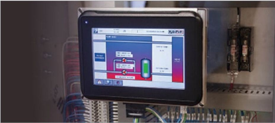
HydroThrift has launched a new advanced industrial control panel.
