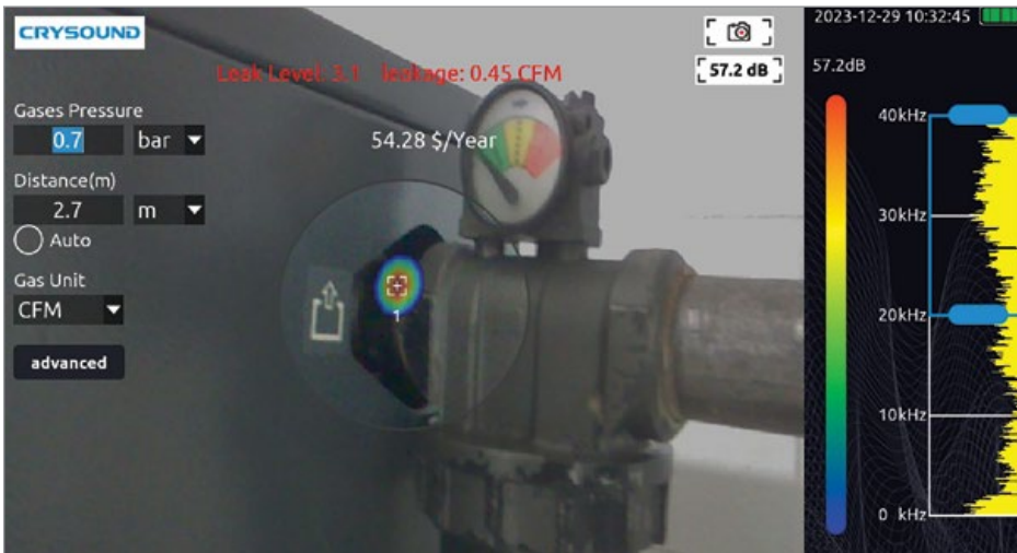
Figure 5: An acoustical imager uncovered leaks, such as this one in the compressed air dryer enclosure.
