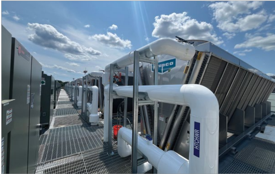
A large-scale cooling installation for a North American data center.
