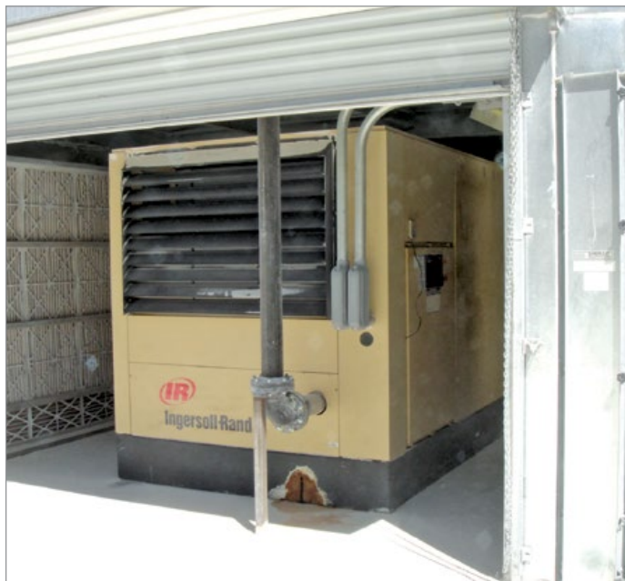
The key to all air compressor technology is to apply it to the right application.
