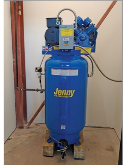
The 5-hp, lubricated, reciprocating air compressor installed at A-1's new Springfield location.
