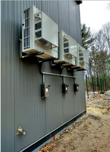
Three condensing units for an air-source heat pump system supporting all of the comfort heating and cooling loads for a wastewater treatment facility in Missouri.
