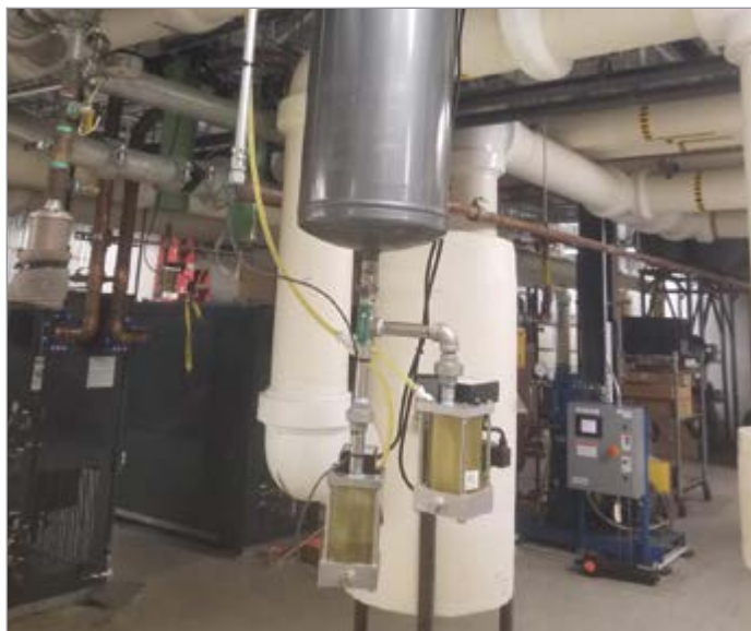
This compressed air system had a centrifugal water separator just after the air compressor. The drain on the centrifugal water separator had failed and was the root cause of the problem.
