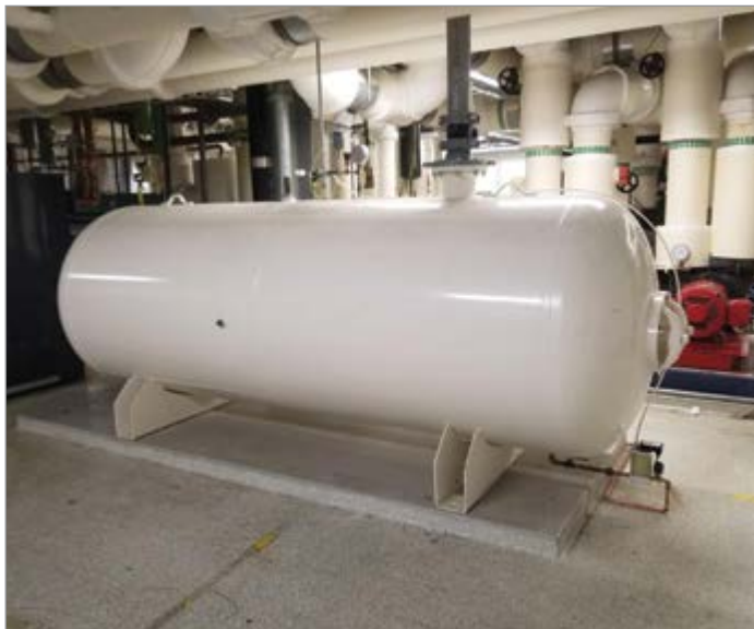
The 1,000-gallon compressed air dry storage tank was almost full of water!
