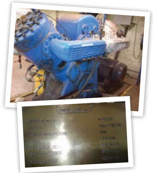
Two subscribers shared pictures from long-running Belliss & Morcom air compressors, one from a South African platinum mine and the other from a Canadian carpet factory.
