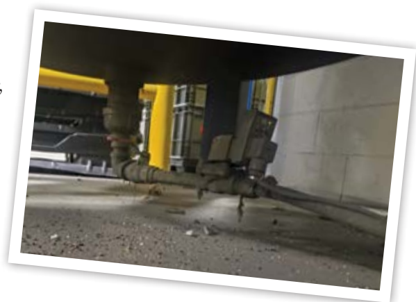
Located under a compressed air storage tank, this timed electric solenoid drain valve presents a challenge for routine plant maintenance.
