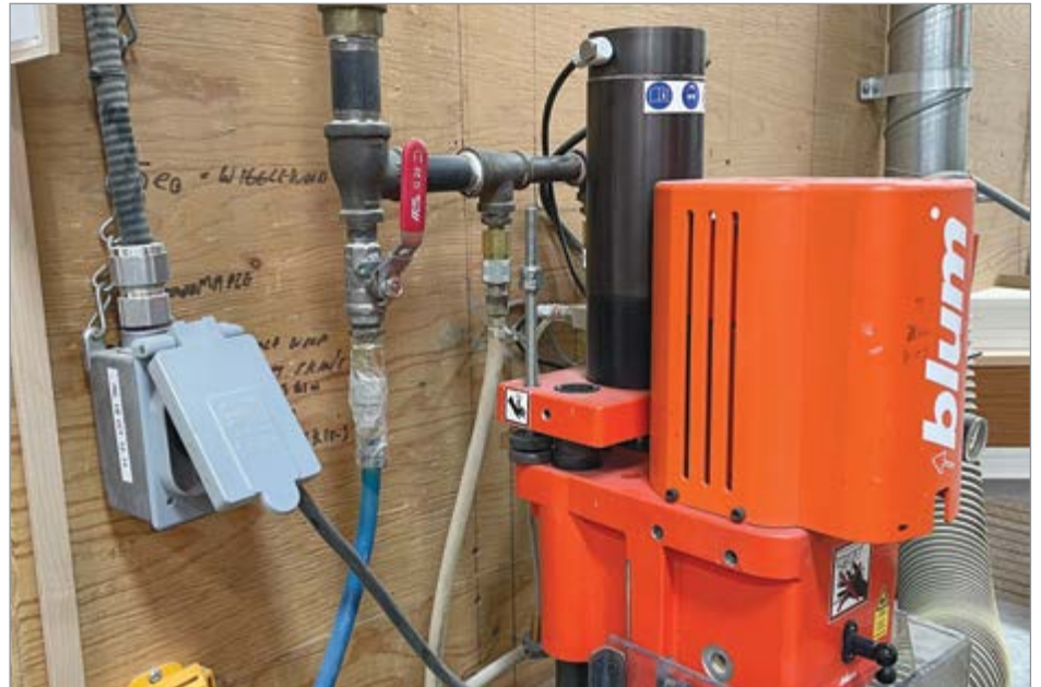
Before working with Air Unlimited, the cabinet maker wrapped this compressed air leak in clear tape.
