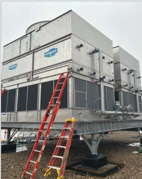
A wireless provider needed a hybrid fluid cooler matching the footprint and weight of its previous cooling tower.
