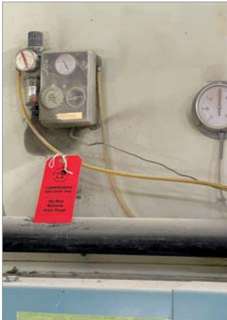
This compressed air leak on the cabinet maker's production line was identified and tagged.
