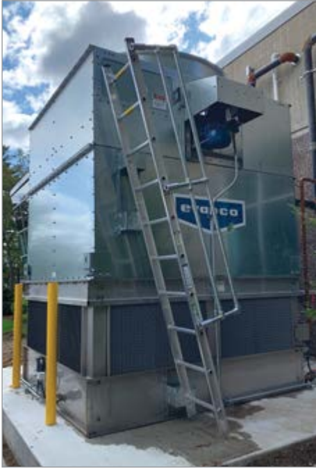
This eco-ATWB hybrid fluid cooler includes a Smart Shield water treatment system, and serves a Massachusetts-based company that does laser powder bed fusion on an industrial scale.
