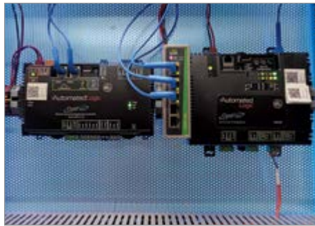
An Automated Logic controller in the central utility plant at Tulane University
