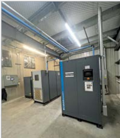
IPS's plan for the Processed Metal Innovators compressor room uses a plenum model to keep the inlet air in an optimal range without a lot of ductwork.
