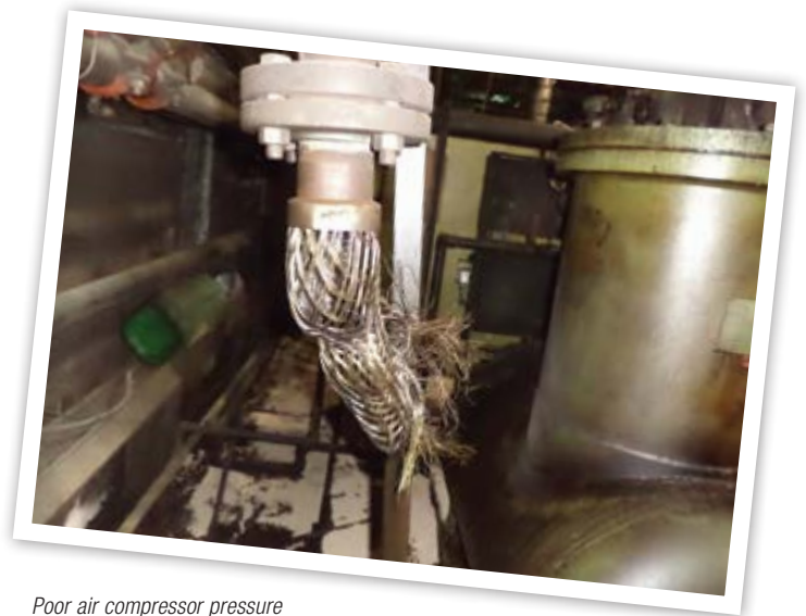
Poor air compressor pressure control caused this flexible connector to fail.
