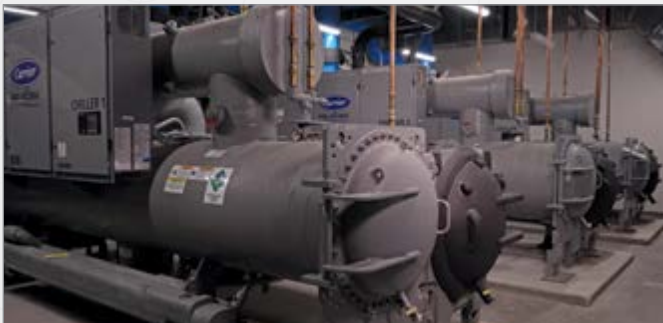
Three centrifugal chillers at Tulane University's central utility plant
