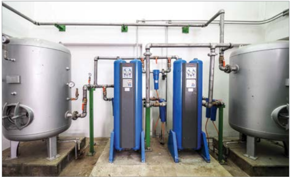
Demonstrate how putting off repairs – such as fixing compressed air leaks – hurts financial performance.
