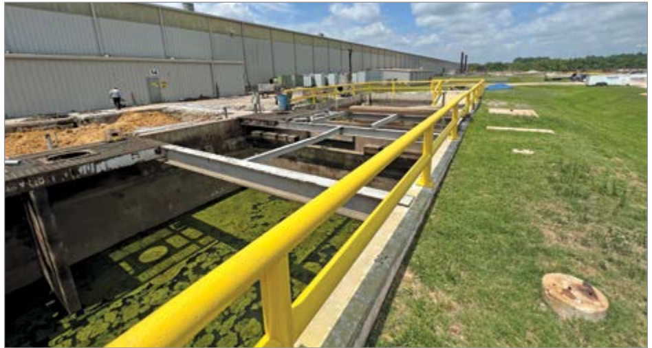
Prior to starting work, the pit was overgrown with algae.
