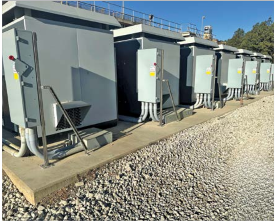
The completed installation of an aeration blower system
