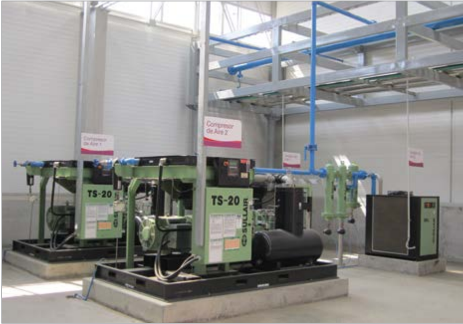
Two tandem air compressors used to make preforms at a plastic bottling plant in Peru.
