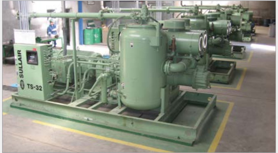
Five tandem air compressors at a Peruvian high-altitude mine.
