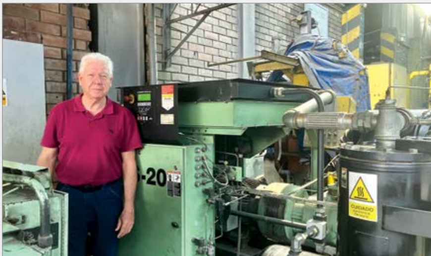
Secada at a tire plant with one of the last Sullair 20-100L air compressors produced.
