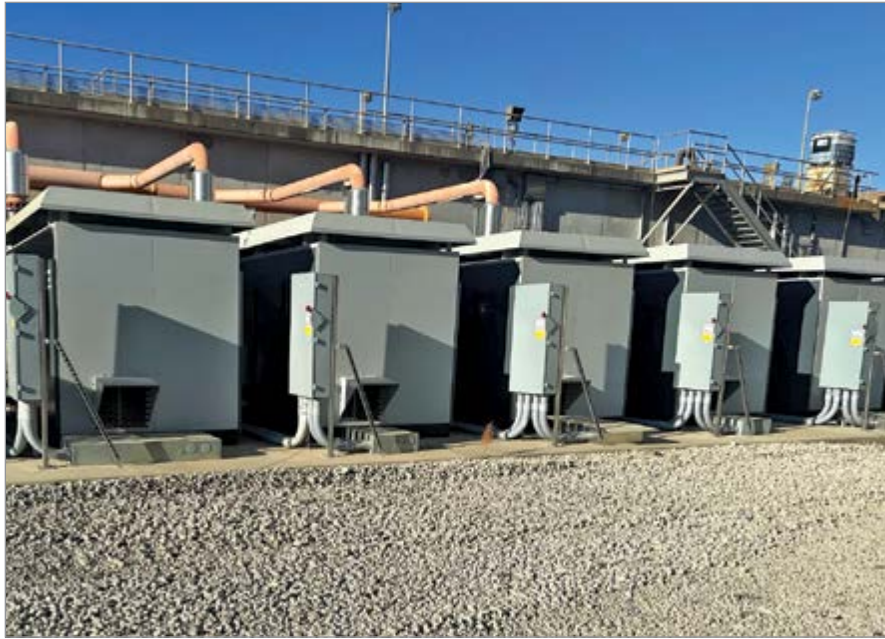
The completed installation of an aeration blower system
