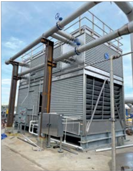
A BAC FXV combined flow cooling tower anchors the closed loop cooling system.
