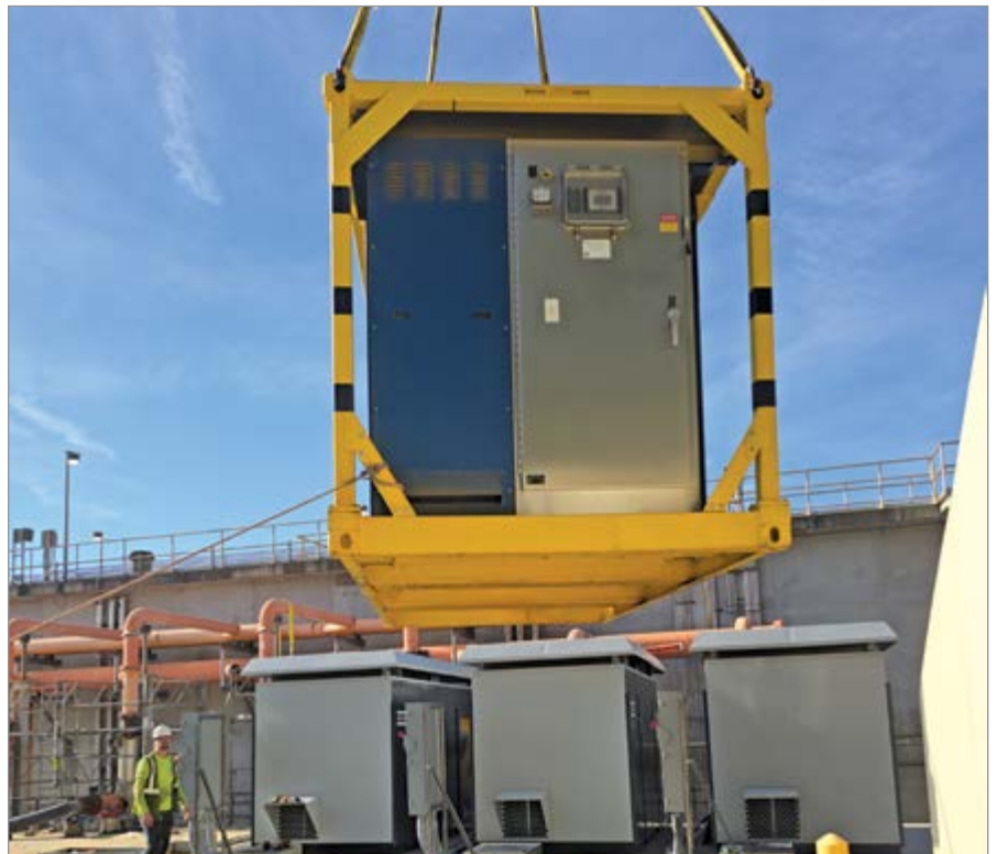
The installation of a high-performance aeration Blower System on a concrete pad
