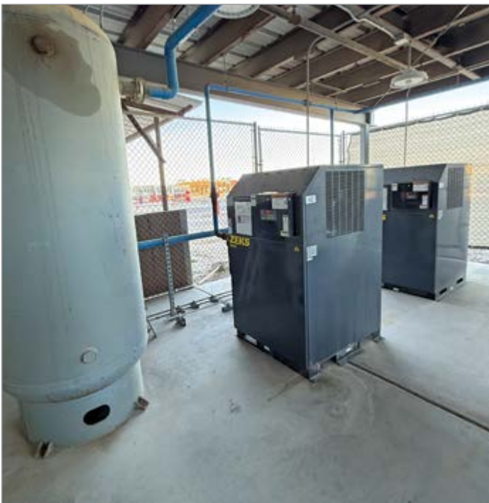
Two properly-sized refrigerated compressed air dryers keep moisture out of the compressed air stream.
