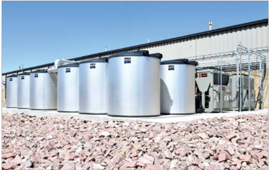
TES tanks installed as part of a thermal battery system outside a manufacturing facility in Pueblo, CO.
