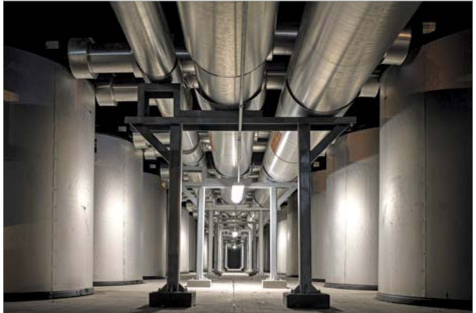
A TES tank installation in the basement of a large commercial building.
