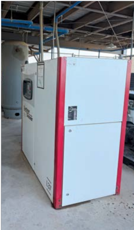
The plant’s compressed air needs are met by a single 50 hp rotary screw air compressor.
