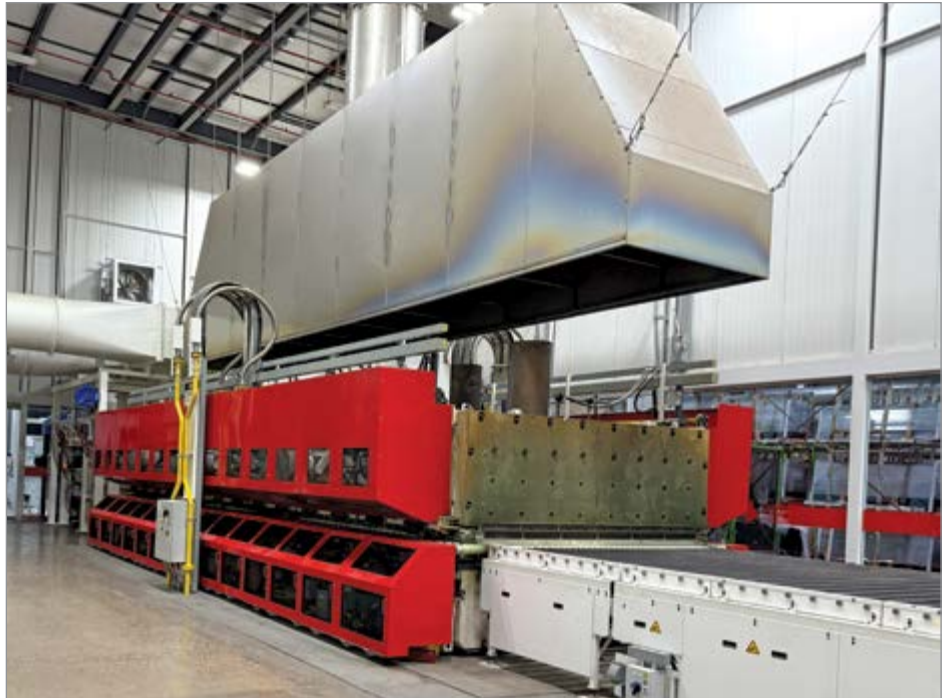
The plant’s tempering furnace reaches 1,250°F (677°C).
