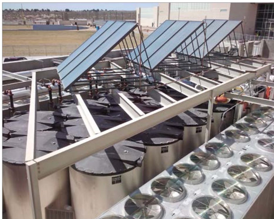
TES tanks integrated with solar panels, supporting renewable energy.
