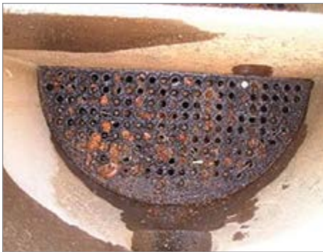
Figure 10. Biofilm on a heat exchanger tube sheet
