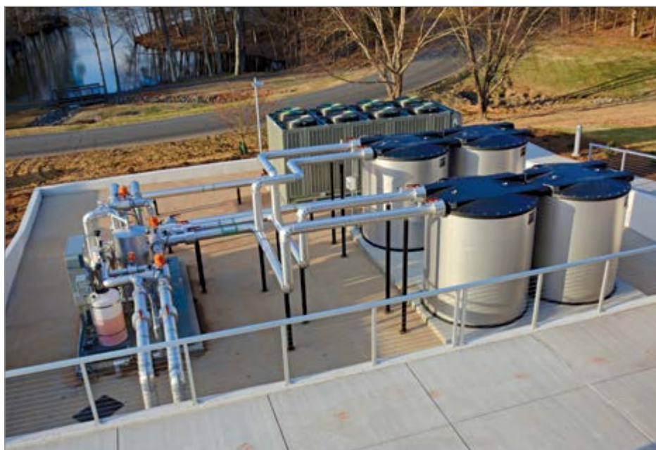
TES tanks installed as part of a thermal battery system outside a commercial building.
