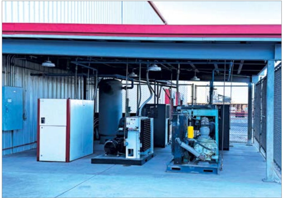
The plant’s compressed air equipment is housed outside under an awning.
