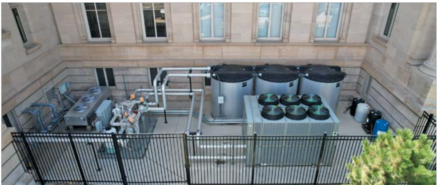
TES tanks installed as part of a thermal battery system outside a manufacturing facility in Pueblo, CO.
