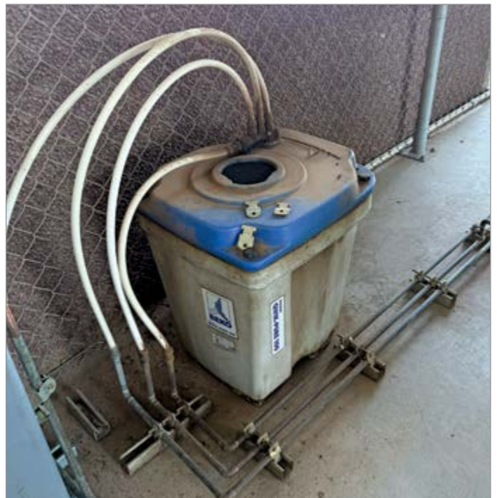
Compressed air condensate now drains into oil-water separators.
