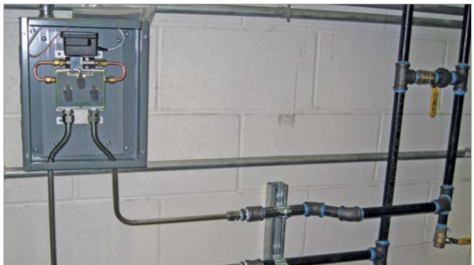
A differential pressure transducer with a three-valve manifold and piped blowdowns
