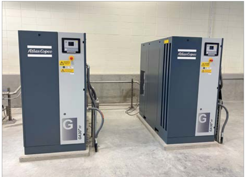
Indoor duty and standby air compressors at a facility in Castle Rock, CO
