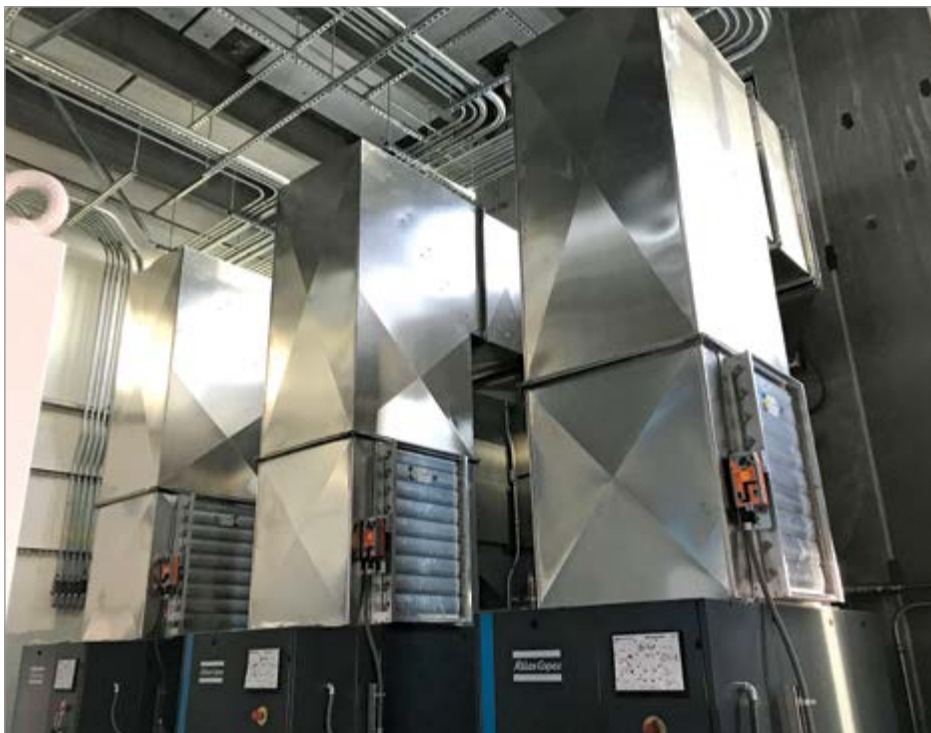
Exhaust ducts solve the issue of heat rejection at a facility in Olympia, WA.
