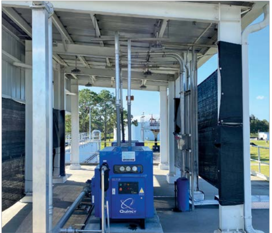
This compressed air system is protected from direct sun and rain at a facility in Orlando, FL.
