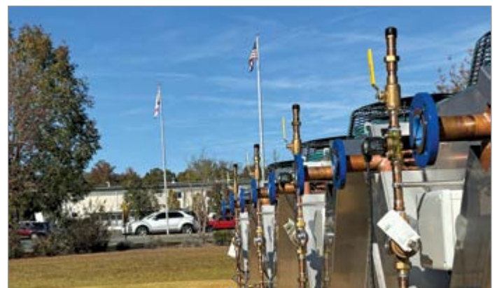
Multiple adiabatic coolers used for trim cooling
