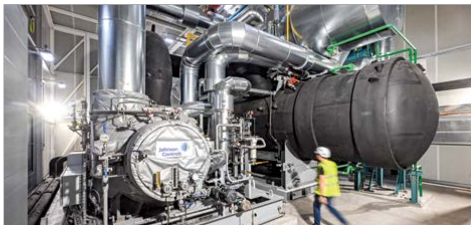
A Johnson Controls large-scale heat pump used for district heating in Southern Germany
