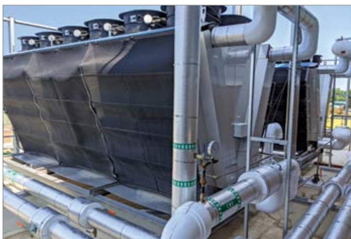
An adiabatic cooler used for chiller support
