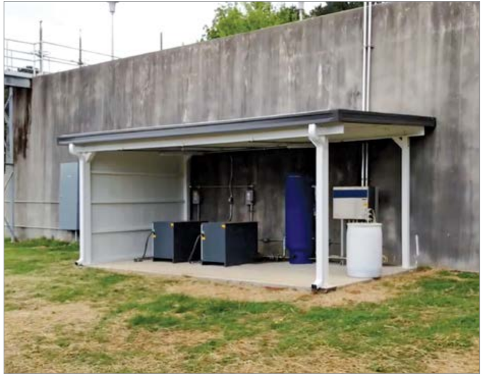
This air compressor, receiver tank and valve module are housed under a tankside canopy in Monroe, NC.
