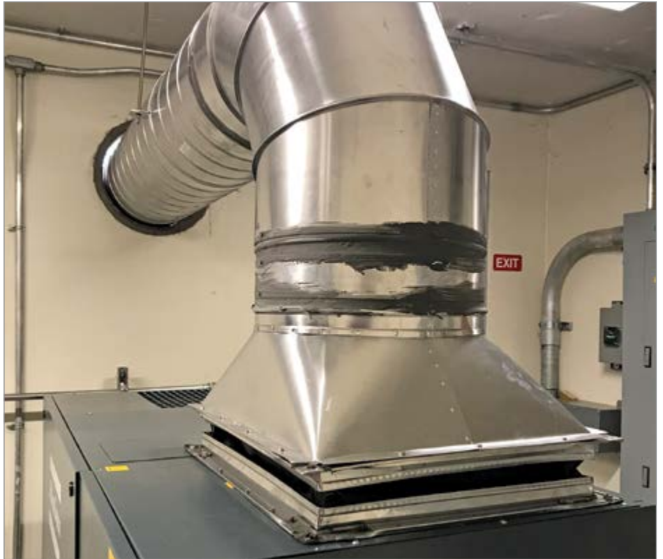
Heat is conveyed out of the air compressor room by an exhaust duct at a facility in Somersworth, NH.
