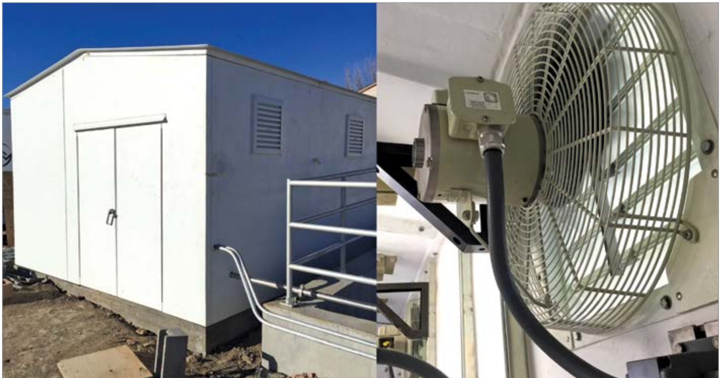
Two exhaust fans are incorporated into an environmental enclosure at a facility in Widefield, CO
