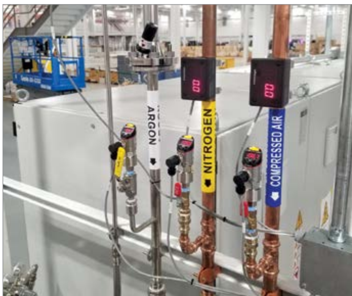
A point-of-use compressed air flow meter and pressure transmitters with displays
