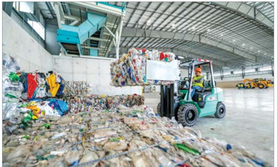
The bundling and packaging system is one of the recycling plant’s compressed air applications.
