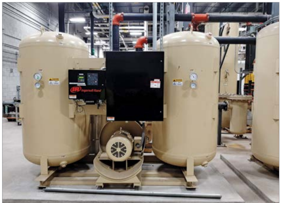
Heated blower purge desiccant compressed air dryers are now standard for all upgrades at Maple Leaf Foods plants.
