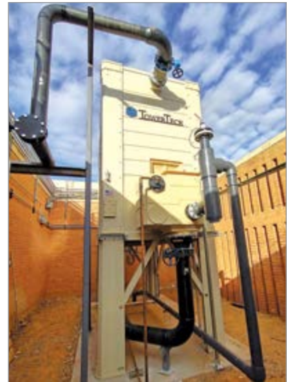
Tower Tech cooling tower installation at a school
