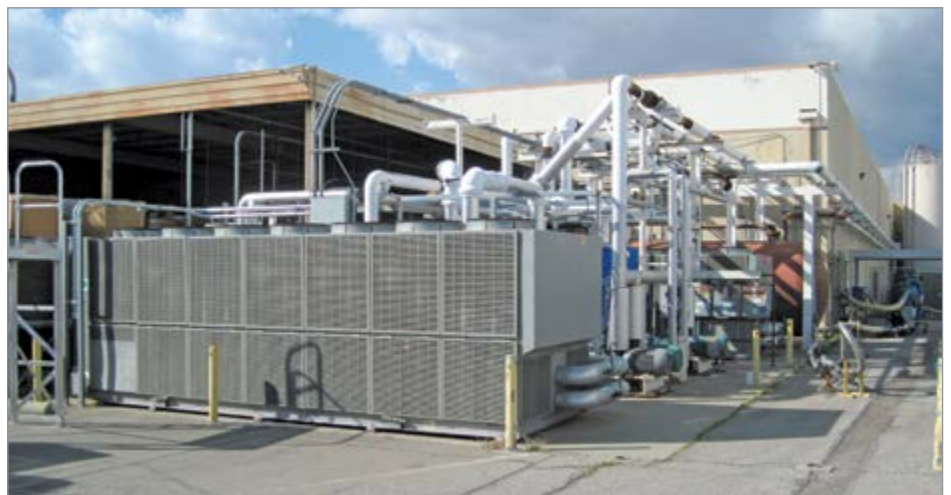
The legacy cooling systems included complicated piping.
