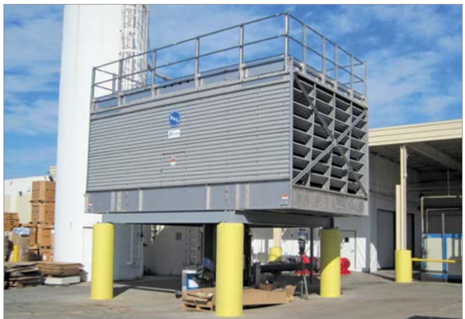
The cooling tower and pumps for the combined cooling system.
