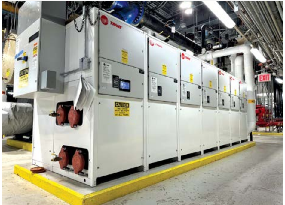
The 55 Water Street electrification retrofit features three banks of Thermafit™ water-cooled, modular heat recovery chiller units, providing heating for the building.
