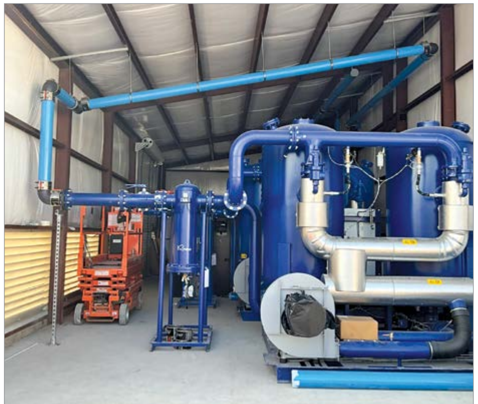
The new air compressor room gives the plant's air compressors and desiccant compressed air dryers a single home separate from other equipment.
