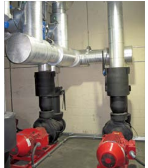
Three-way valves and dedicated pumps enable the combined cooling system to meet distinct cooling criteria.
