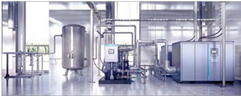
A heat of compression, rotary drum compressed air dryer and an oil-free rotary screw air compressor
