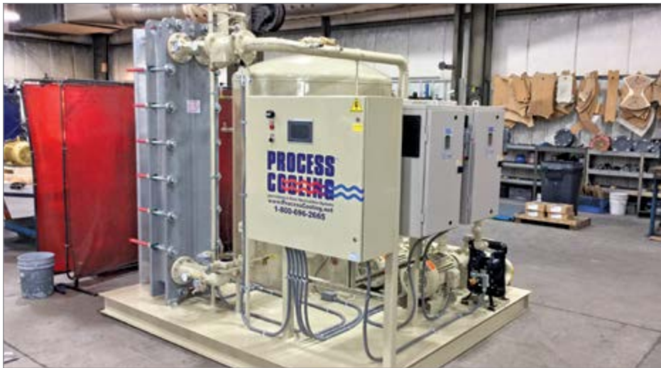
This closed-loop assembly was built for a heat treating facility in New Hampshire. It includes plate and frame heat exchangers and a tank with a nitrogen blanket. A nitrogen-driven pump offers security in case of power loss.
