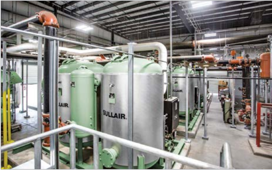
A heat of compression dryer installation
