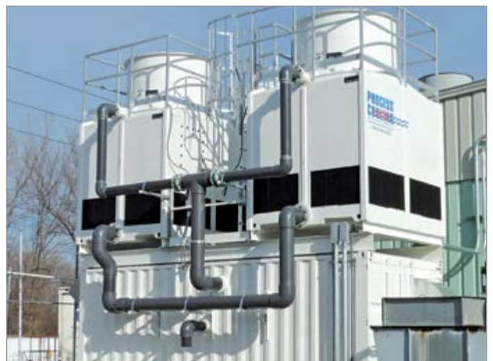
This modular mechanical room with cooling towers built into the structure was built for a heat treating application in New York.
