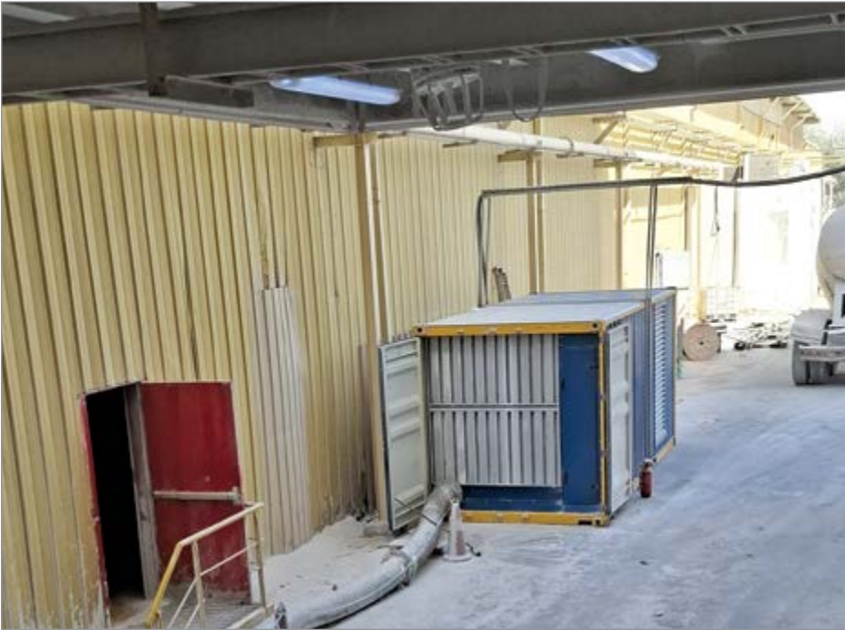
A gypsum plant in Saudi Arabia used a rental air compressor while waiting on purchased air compressors that would be permanently installed.
