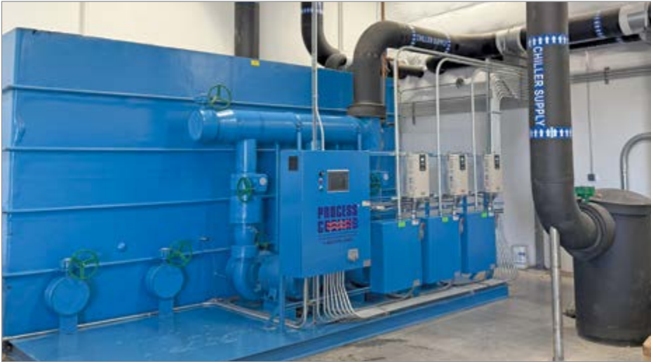
This chilled water pump and tank assembly at a plastic injection molding facility in Arizona has a 5,300-gallon capacity with provisions for pump expansion in the future.
