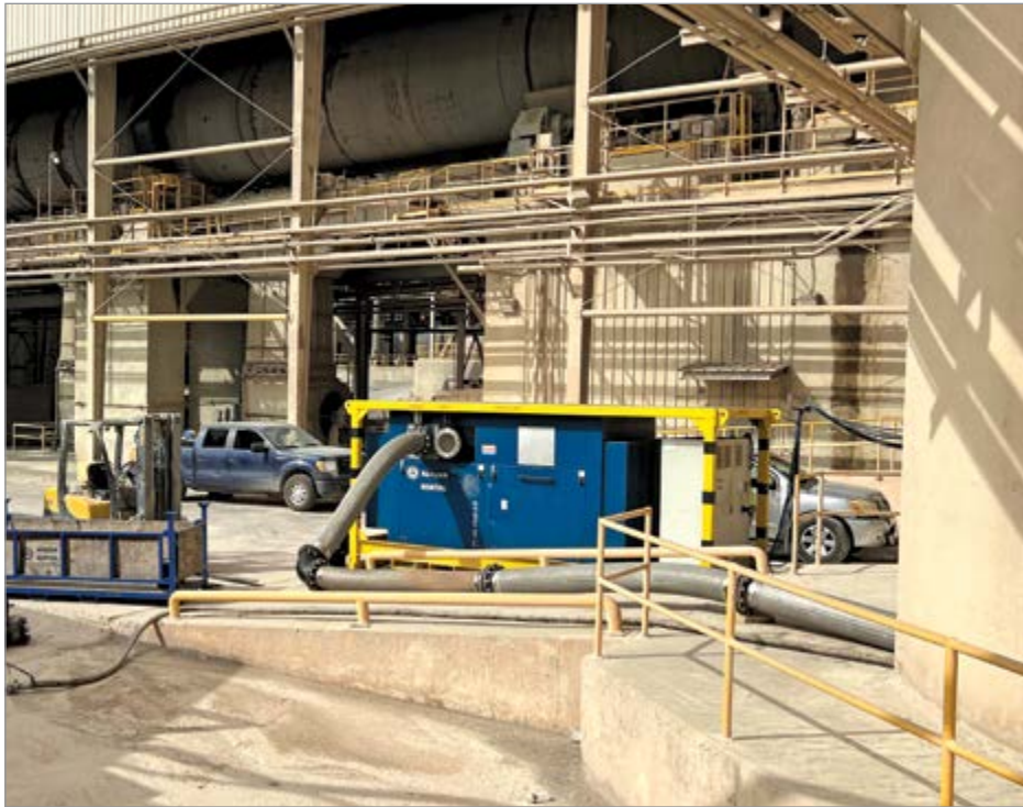
A cement plant in Texas relied on a rented industrial blower to replace a rented diesel air compressor while awaiting permanently installed units.
