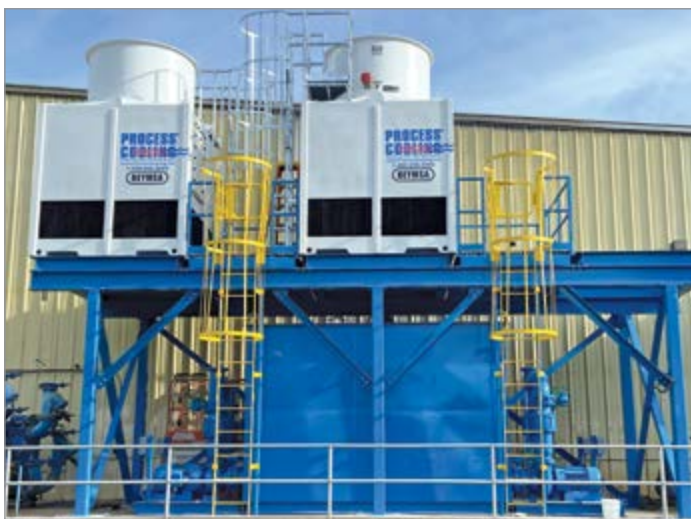
This central cooling tower system was built for an all-outdoor installation in North Carolina.
