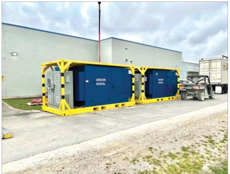
These rental air compressors were used temporarily while permanently installed air compressors were on order.
