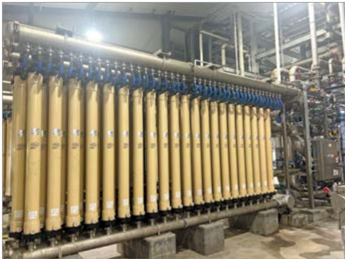
The water treatment plant uses two levels of filtration. The first is a microfiltration system that removes total suspended solids.
