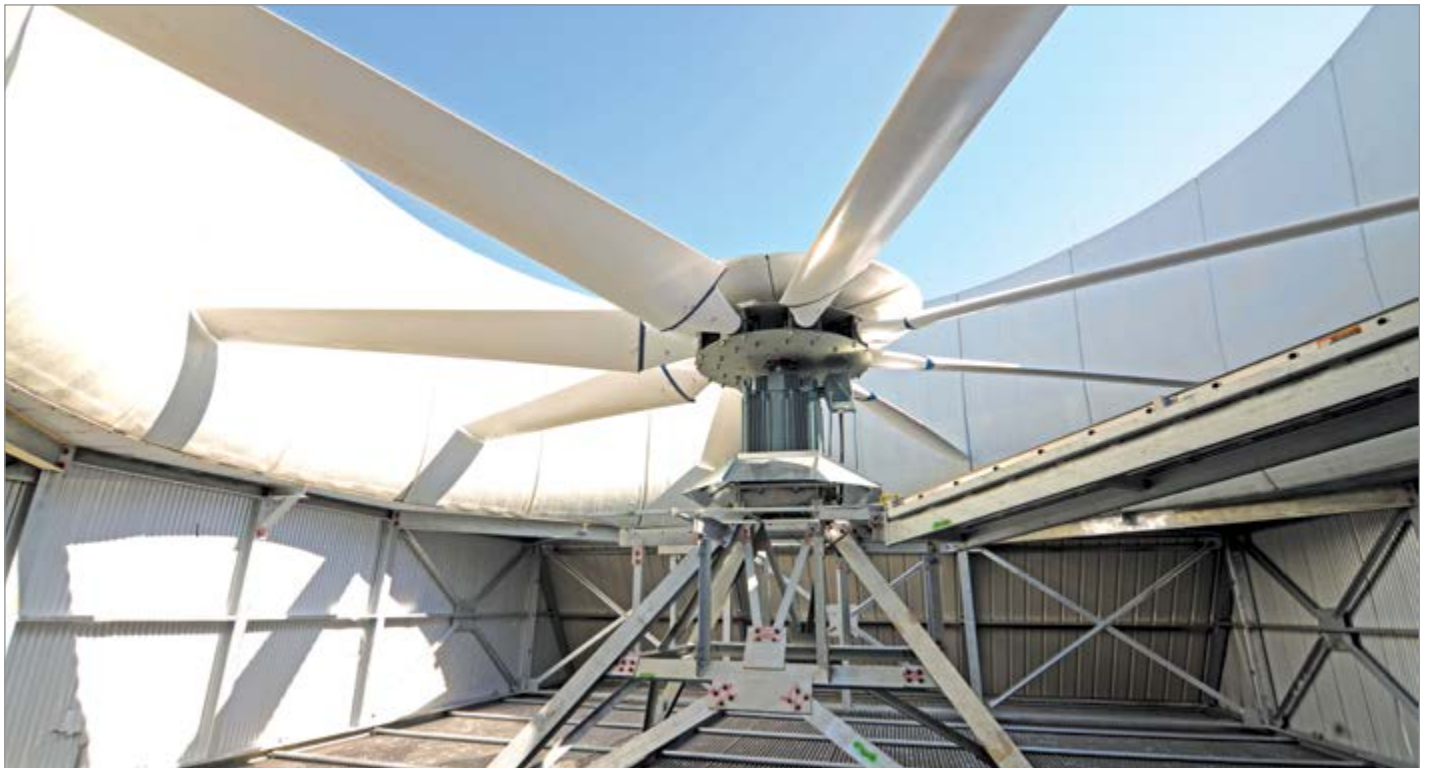
Direct drive motors improve cooling tower energy efficiency and system cleanliness, while reducing maintenance.
