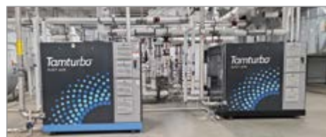
This oil-free centrifugal compressed air system is one of Gentex's 15 compressed air systems.
