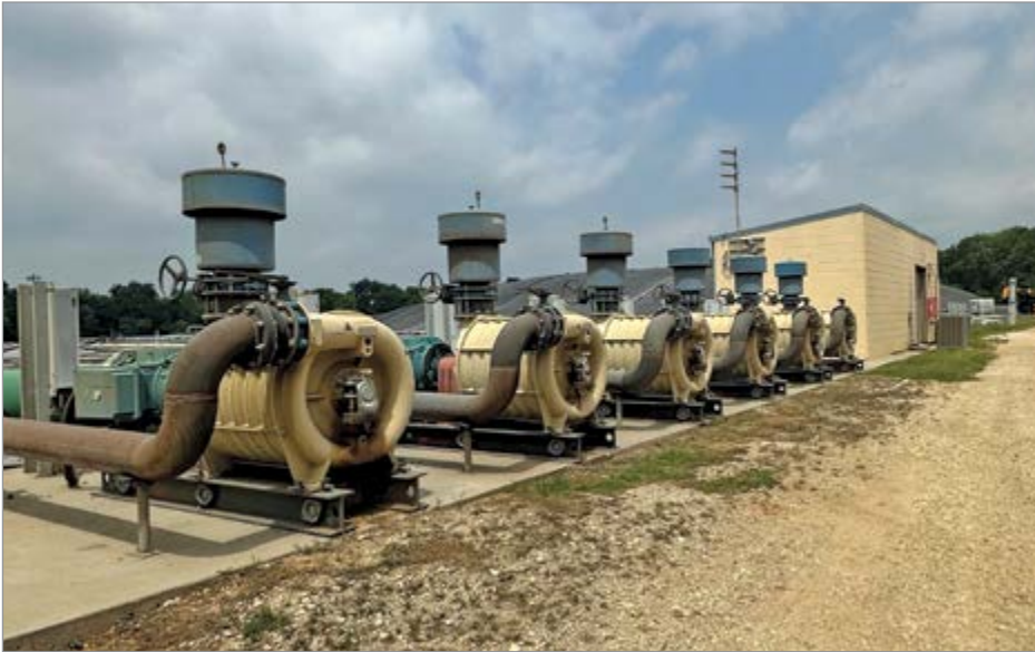
These multi-stage centrifugal blowers are permanently installed and owned by a water treatment plant in Texas.
