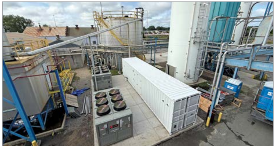
Located at an asphalt shingle facility in Minnesota, these air-cooled chillers each provide 60 tons of cooling.
