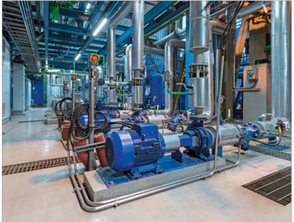
To address underlying system issues, a pump system assessment looks at the system as a whole, rather than treating each component in isolation.
