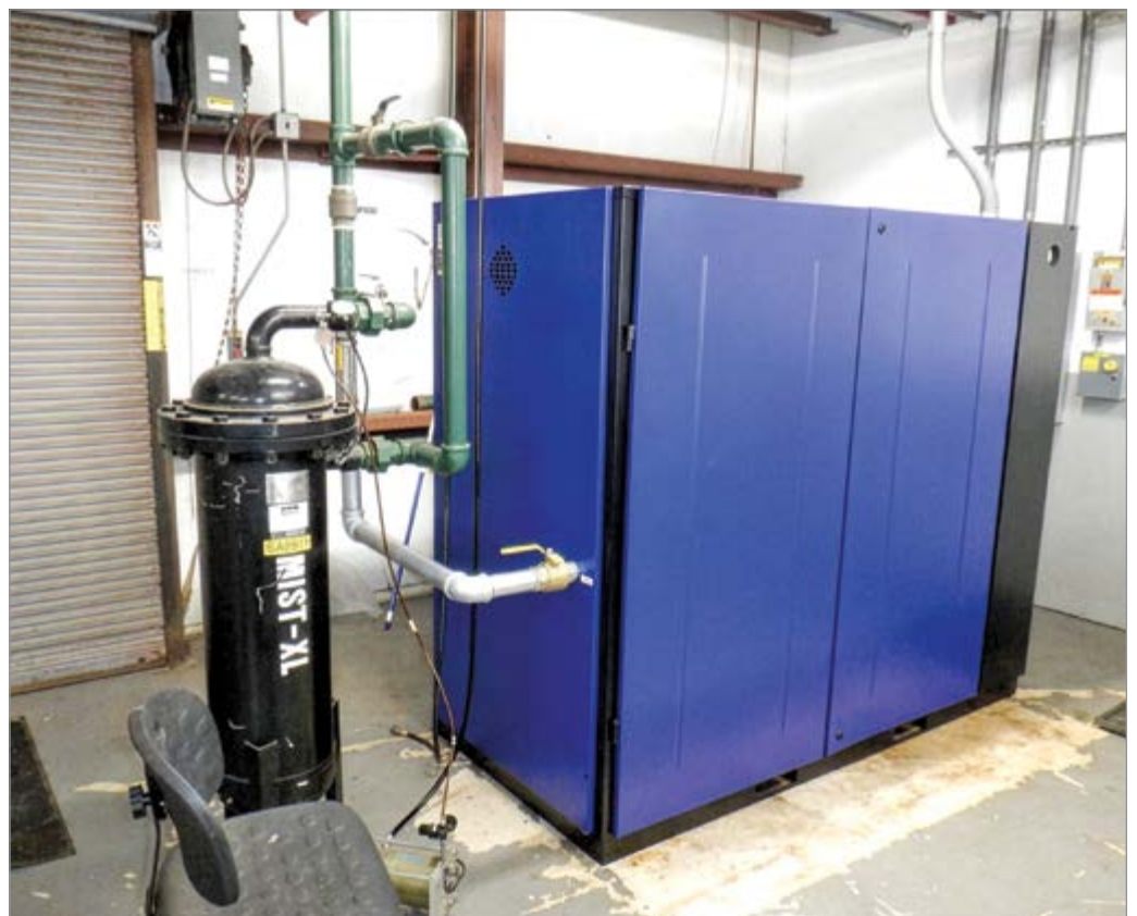
The company installed a 75 hp, variable-speed, lubricated, air-cooled, rotary screw air compressor.
