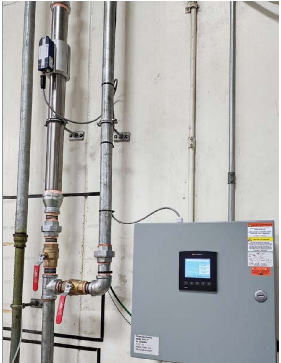
An inline flow meter was used at the Canadian factory.
