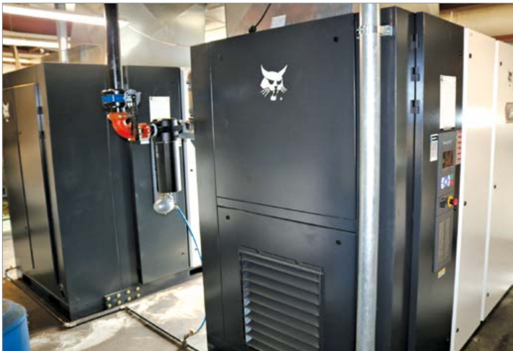
Riley chose to replace the previous VSD air compressor with smaller VSD and fixed-speed air compressors.
