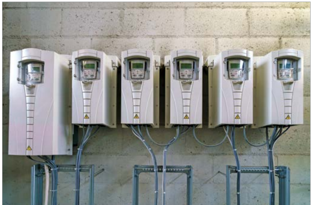
In a high-rise building, converting chilled water pumps to variable speed operation and implementing demand-based control can cut energy use while improving occupant comfort.
