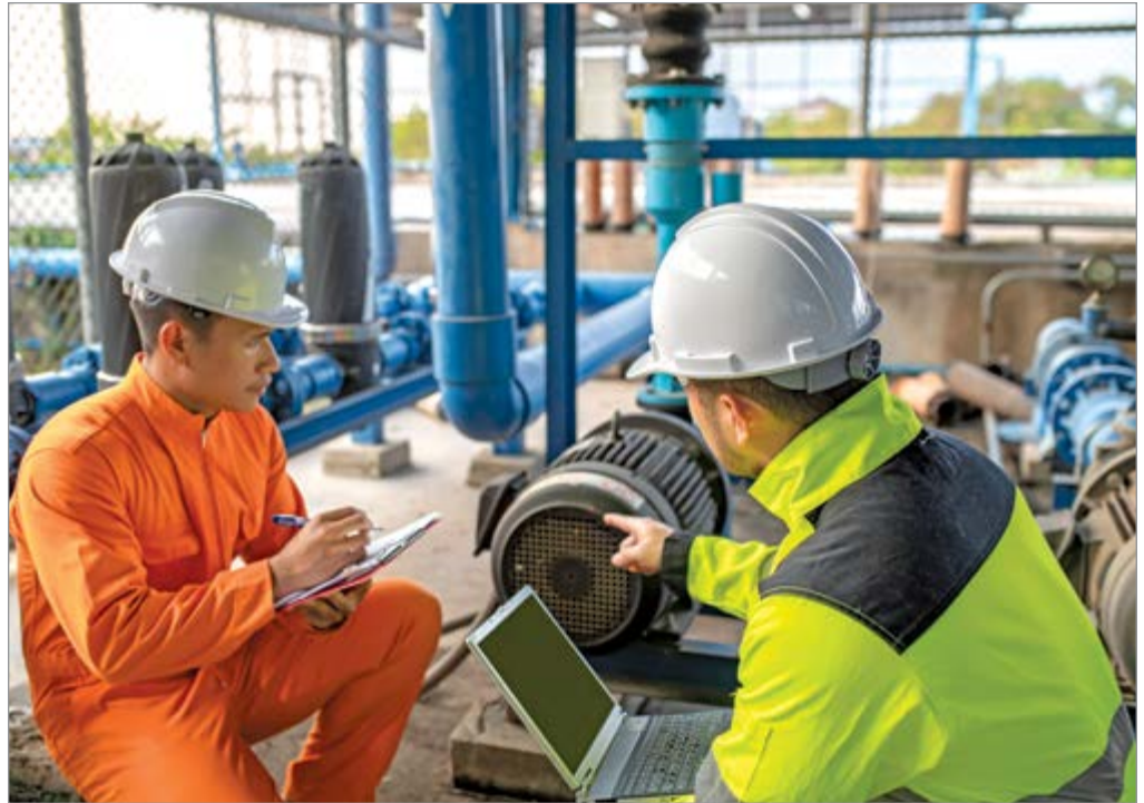
Assessment teams include operations and maintenance staff who are familiar with the pump systems and how they are run, engineers who know the design intent and, ideally, a PSAP-certified professional.
