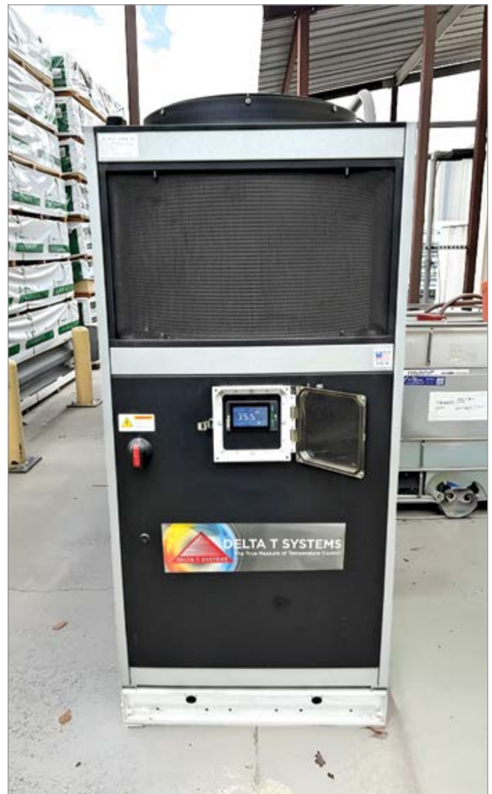
Delta T Systems modified the controller on this chiller so the customer can chill water 25°F (14°C) below the ambient dew point.
