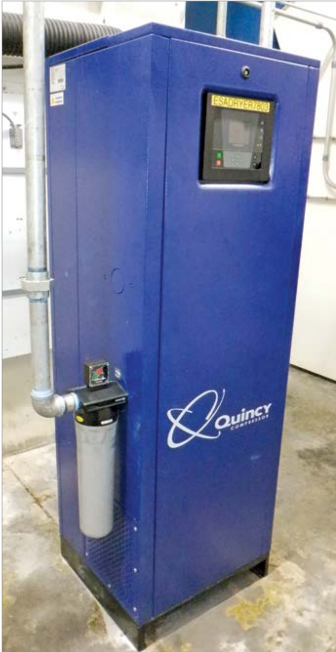
A new heatless desiccant compressed air dryer solved the problem of too much moisture in the compressed air stream.
