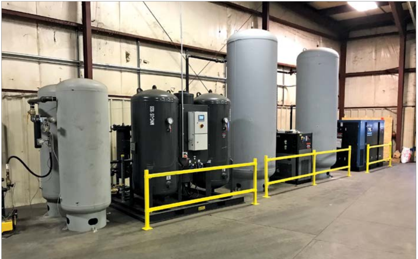
This complete nitrogen generation system includes an air compressor, wet and dry compressed air storage tanks, a refrigerated compressed air dryer, a PSA nitrogen generator and a nitrogen gas storage tank.
