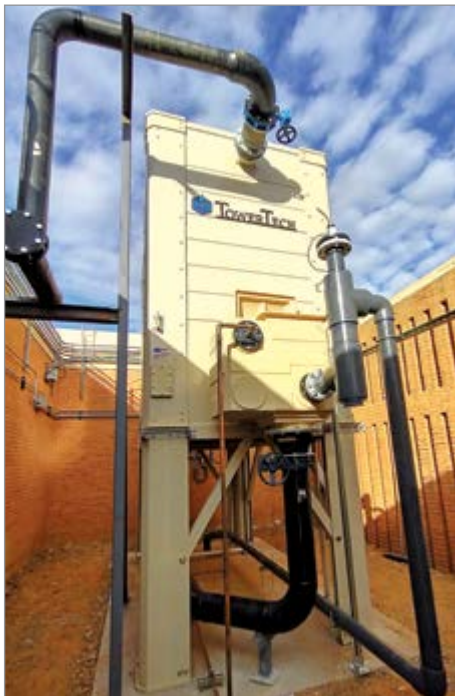
A Tower Tech StormStrong 100-ton cooling tower installed at a school
