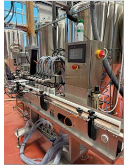
The brewery's canning line is powered by compressed air.
