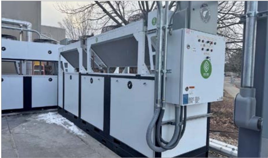
The Elite 290 propane chiller was installed at New Belgium Brewing.
