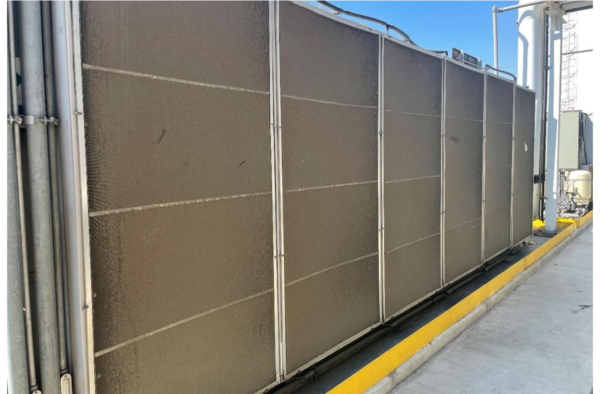
Chiller coil screen – L.A. Basin location
